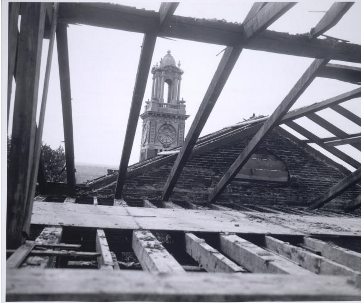
FIGURE 2.20. Hope College roof during 1958 reconstruction. Photograph, facing west (Carrie Tower in the background), 1958.
